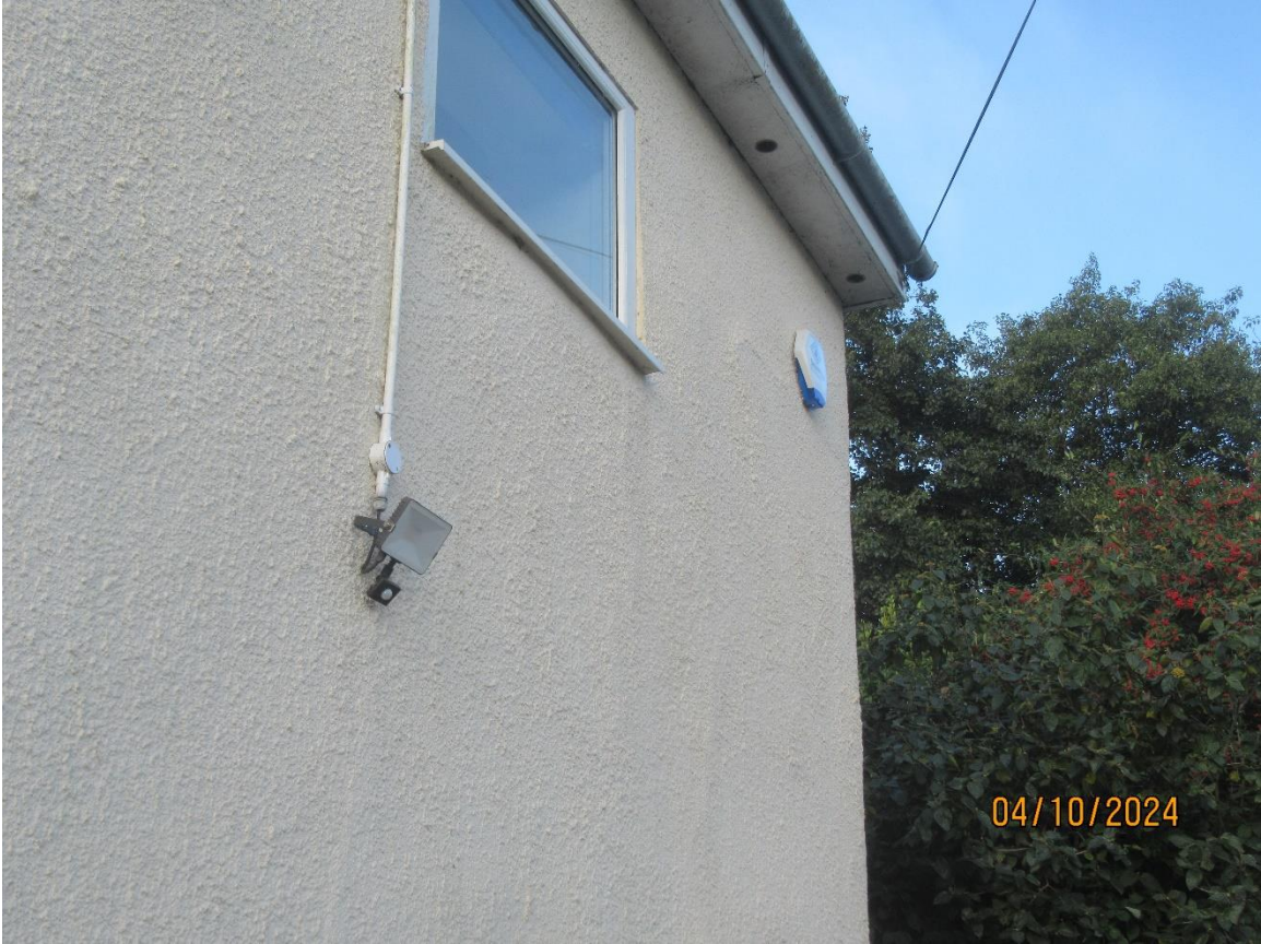
P13 – depot bulging wall
