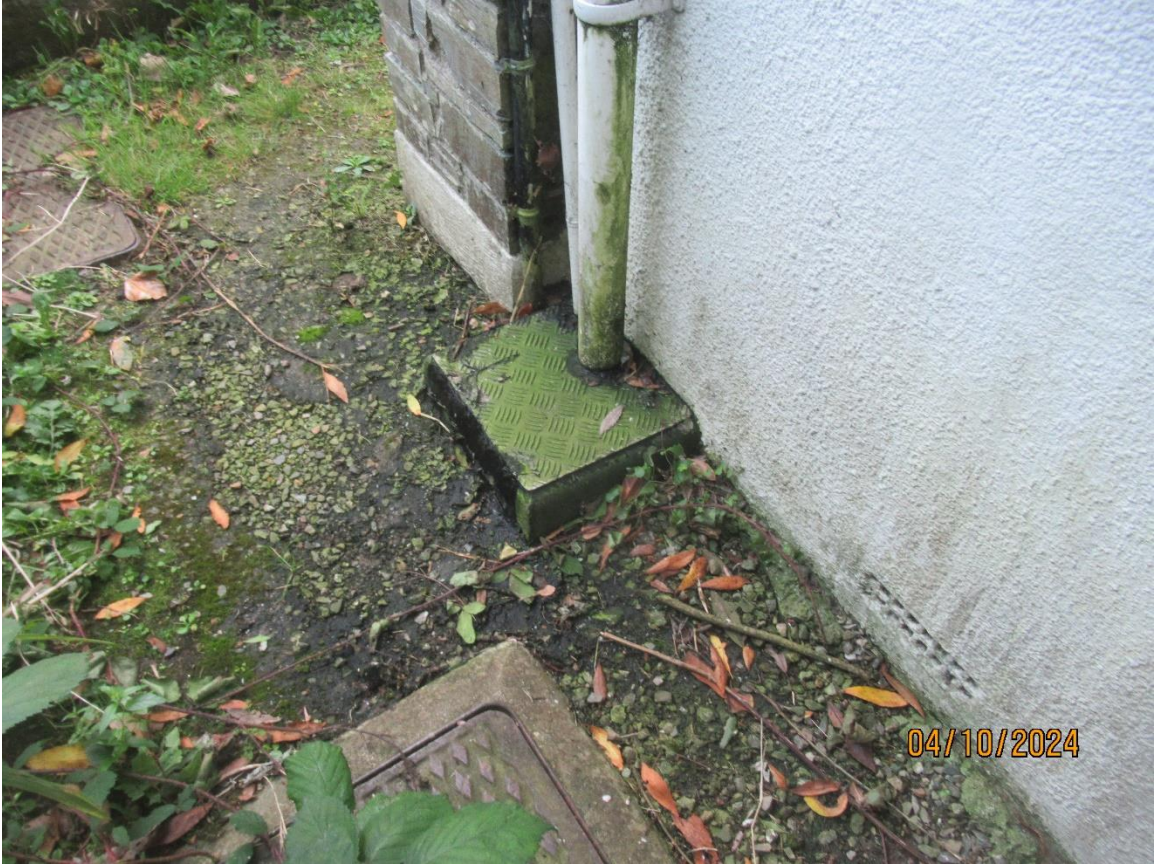
P7 – Maurice Huggins mossy downpipe
